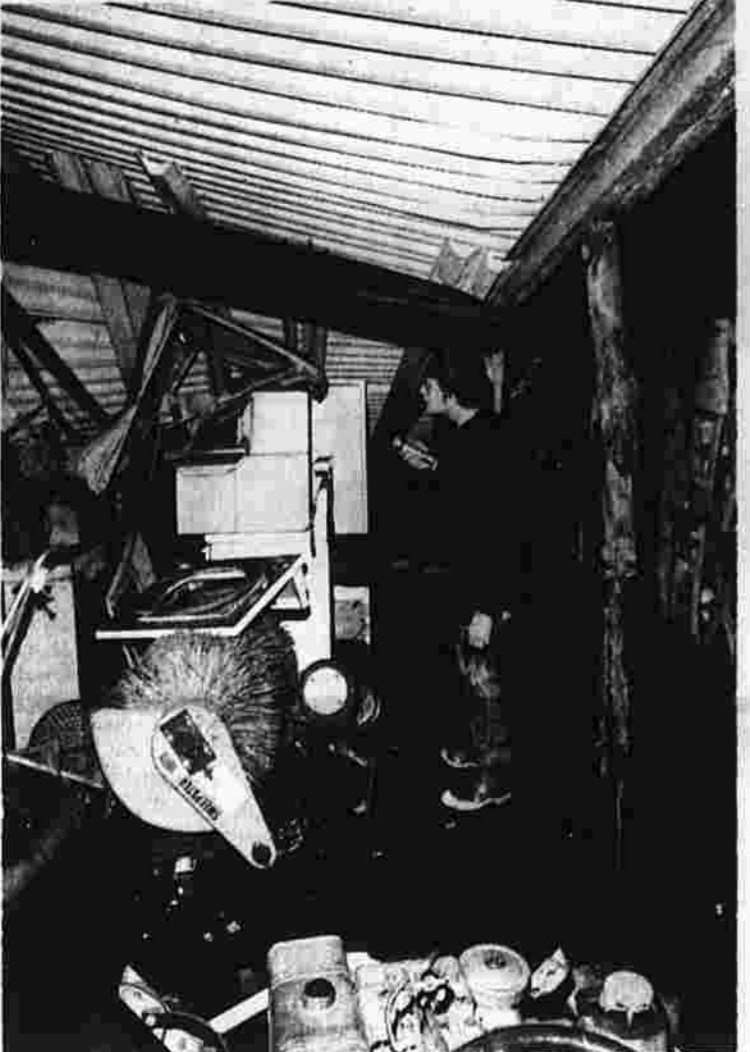
Storm damage in Bolton A storage building at W. J. Preuss, Rt. 44A in Bolton was one of last week's victims of the snow and ice storm. The outside of the building looked like a mini version of the coliseum roof collapse at the Hartford Civic Center. Shown inspecting the sagging beams inside is Jim Preuss Jr. (Herald photo by Dunn)
